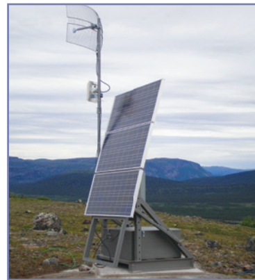
Figure 3: stand-alone remote data-acquisition station equipped with GPS, solar power and radio transmission. Paladin data loggers are housed within NEMA-4 junction boxes at the base of the unit
