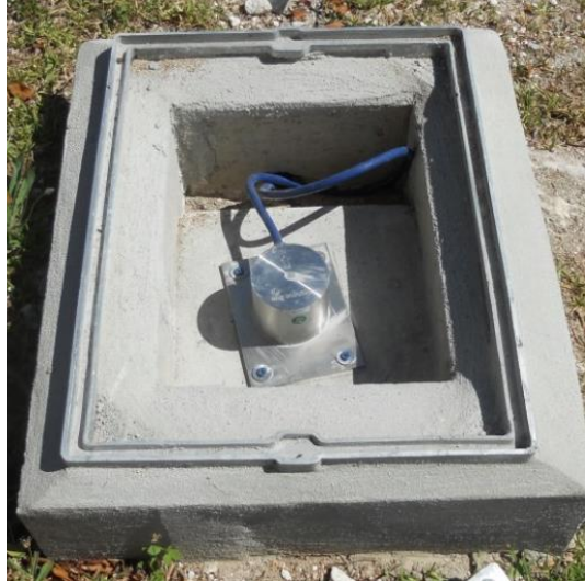
Figure 1 The FBA sensor installed in its purpose built enclosure. The cable is installed at shallow depth to ensure the cable is not accidentally interfered with.
